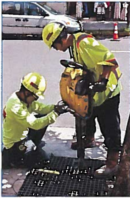
A sleeve for a new sign post is installed to designate where the three minute passenger loading zone begins.
