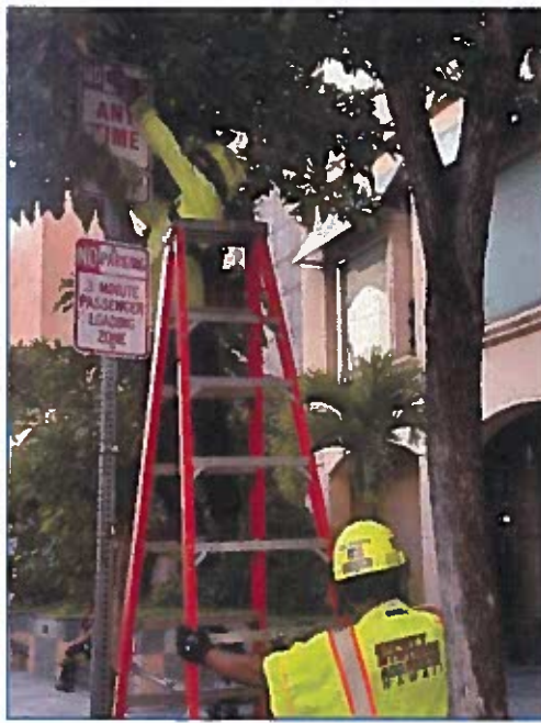
The new three minute passenger loading zone sign has been installed and the old "NO PARKING ANYTIME" sign is being removed.
