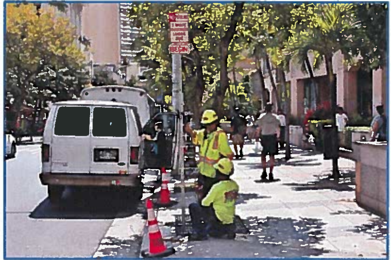
The first new sign is installed on a new post to establish the beginning of the expanded 365-foot long three minute passenger loading zone.
